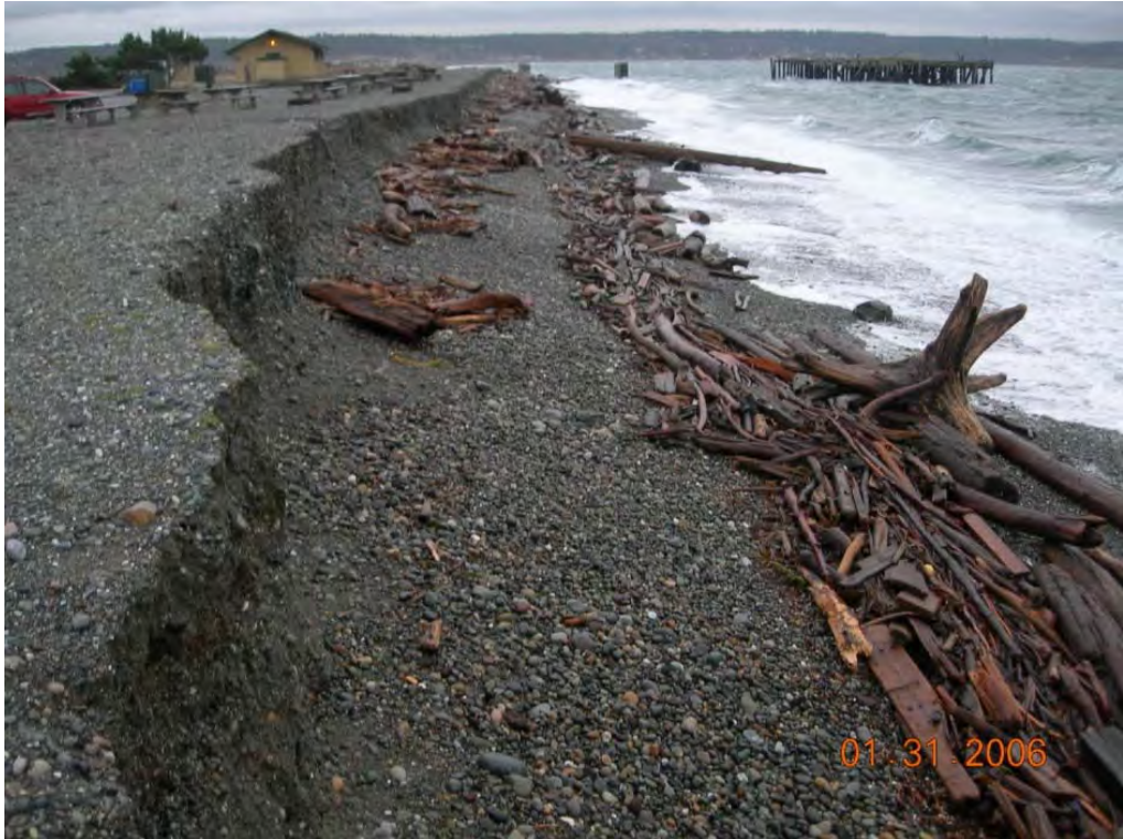
Figure 24. Dredged material disposal area for beach nourishment to protect park infrastructure at risk of damage from shoreline erosion.
