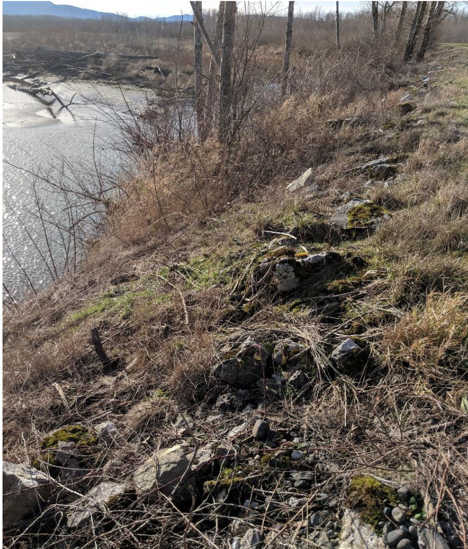
Typical levee condition upstream of the scoured area. The riverward toe of the levee is steep due to missing riprap.
