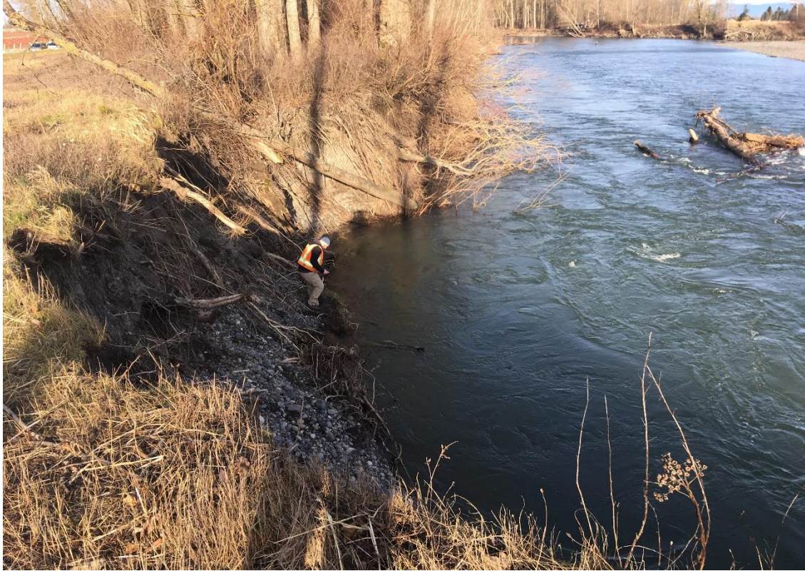
Near vertical bank from scour pool.
