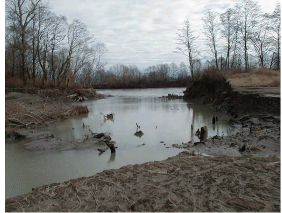
Figure 6.1, Levee breach in Lynden, WA (NWS)
