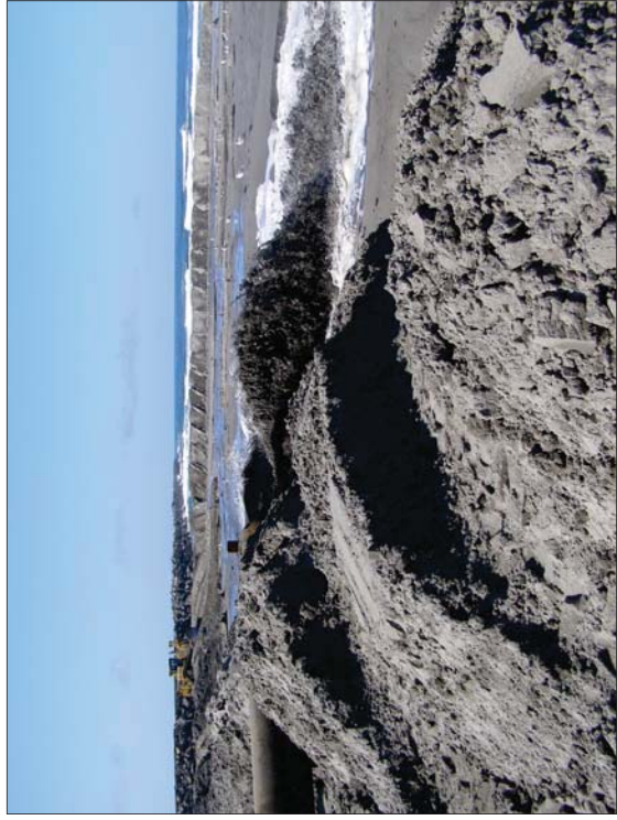
Direct beach pump ashore from a hopper dredge via a floating pipeline (over North Jetty of Columbia River onto Benson Beach, 2008). Note sand berms to contain material.
