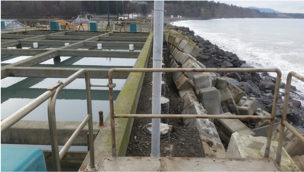
Figure 3. Section in front of paper mill filtration pond damaged in the December 2015 storm (prior to emergency repair).
