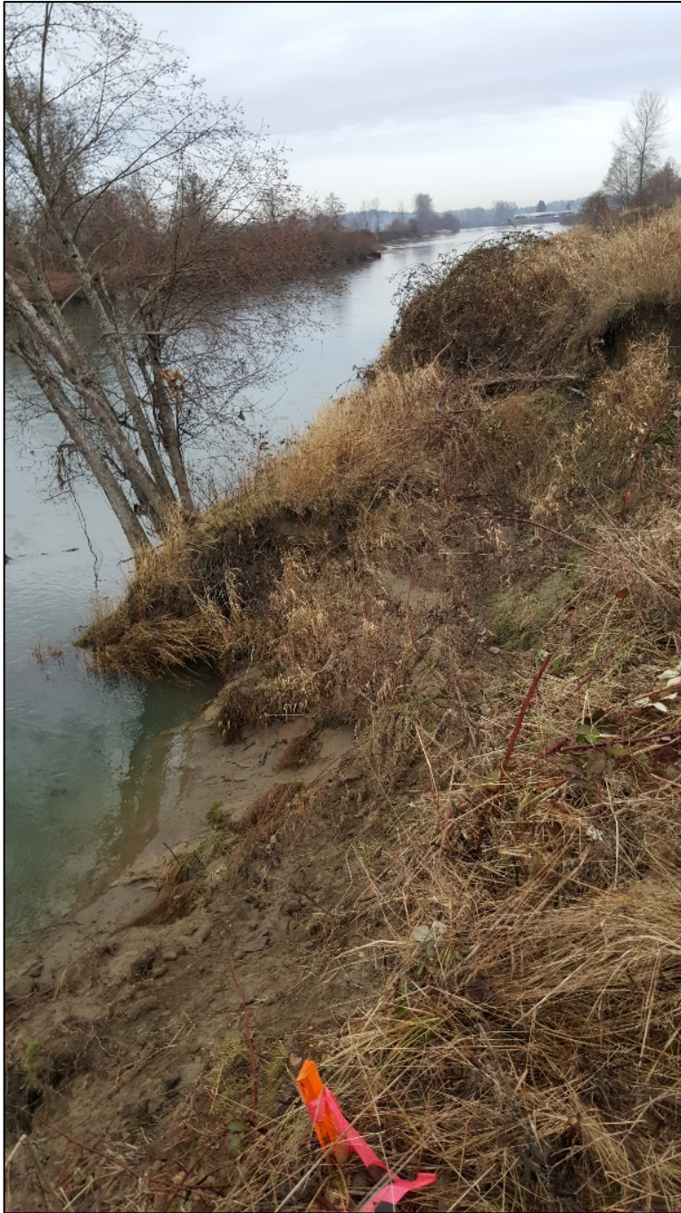
Photo 1. Lord Hill site looking downstream towards the damaged area.
