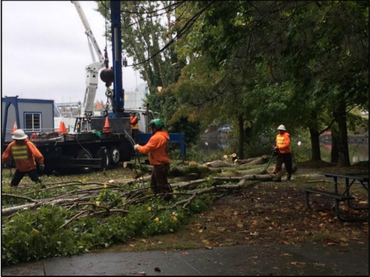
Figure 17. Poplars that line Fremont Cut are in Phase III (2018) of a four-phase removal and replacement plan.
