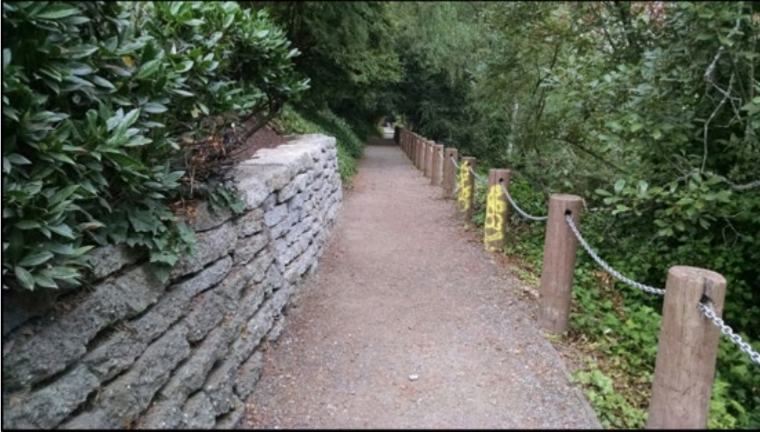
Figure 42. Montlake Cut Waterside trail showing a completed repair of a portion of a stone wall in 2018.
