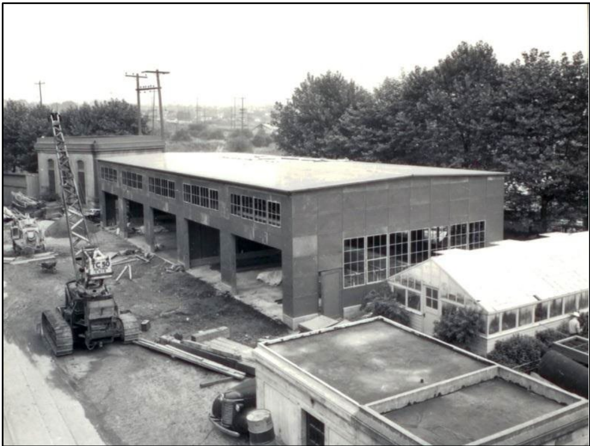
Figure 35. Construction of the steel shop in 1941. Note greenhouse at right of the shop.
