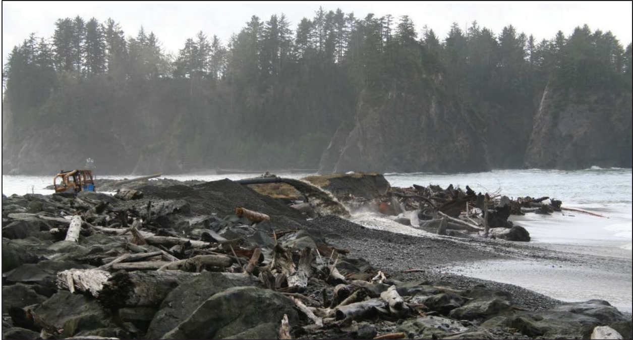
Figure 1. Site B looking west; bulldozer on riverside of Quillayute Spit with pipeline and sediment placement on the ocean side of the spit.
