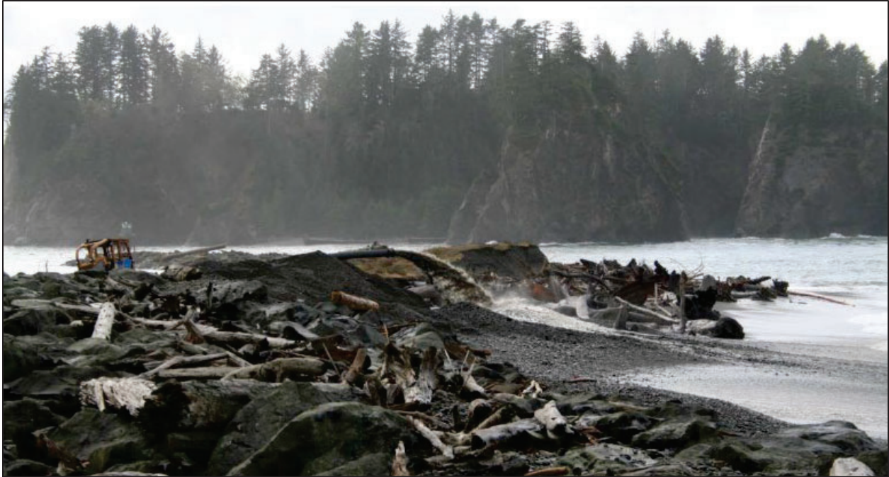
Figure 4. Site B looking west. Bulldozer on riverside of Quillayute Spit with pipeline and sediment placement on the ocean side of the spit.
